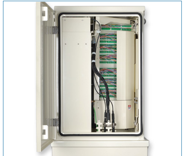
OptiTect Local Convergence Cabinet, LS Series, 432-Fiber (rear door removed) | Photo FOH354
